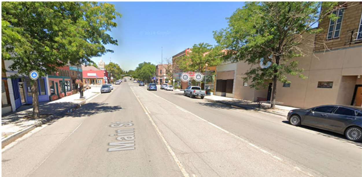
Figure 3-9. Condition of Striping on Main Street
